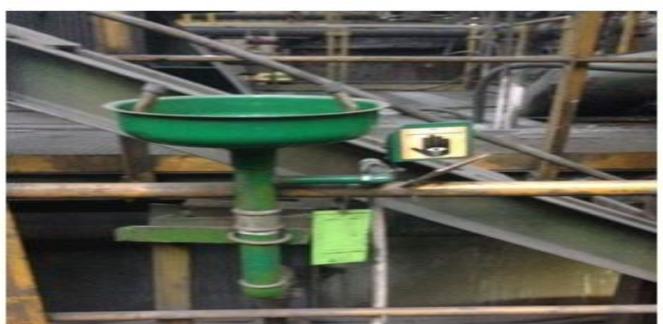
Figure.6. Eye washing station (Helvacioğlu, 2016).
